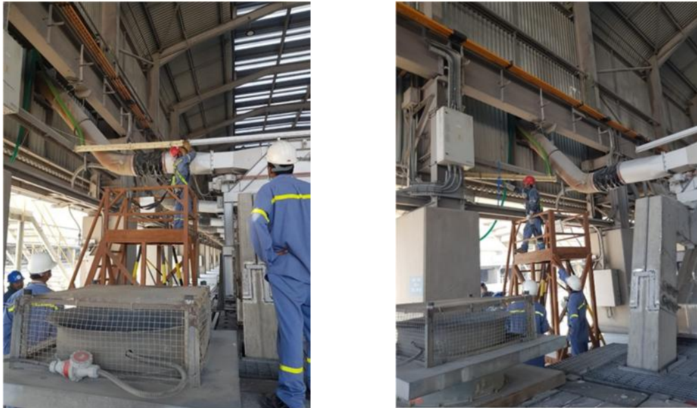
Figure 5. Left: installation of crossover/transport air slides; Right: installation of crossover/transport air slides.
